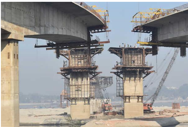
The Guwahati-North Guwahati bridge over Brahmaputra when it was in construction in November 2023
